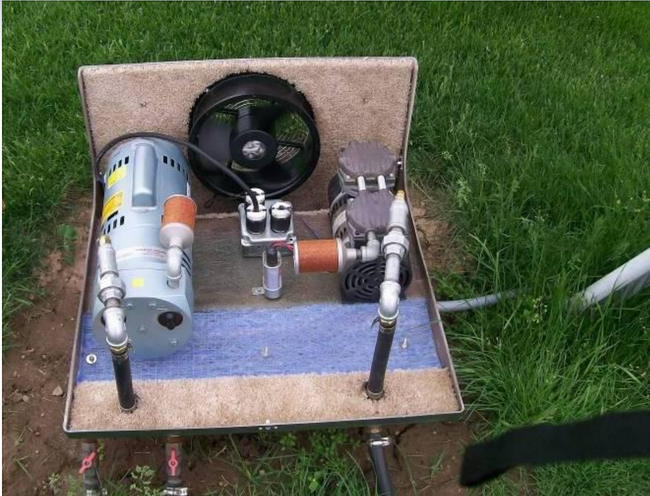
Inside of a compressor cabinet after one year in operation under Lake Savers Management Program
